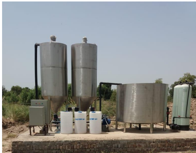
Figure 1: Wastewater Treatment Plant at the KFUEIT
