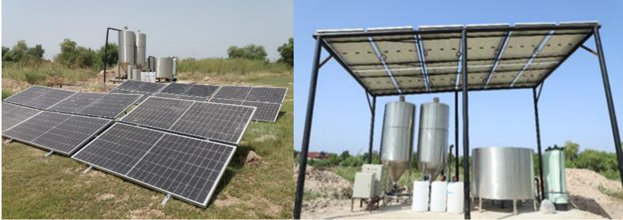
Figure 2: Solar Assisted Wastewater Treatment Plant
